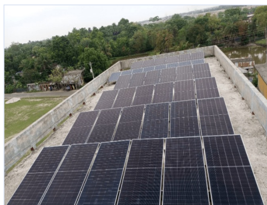
Figure: Solar Panels of 1st Adaptation Fortress rooftop
